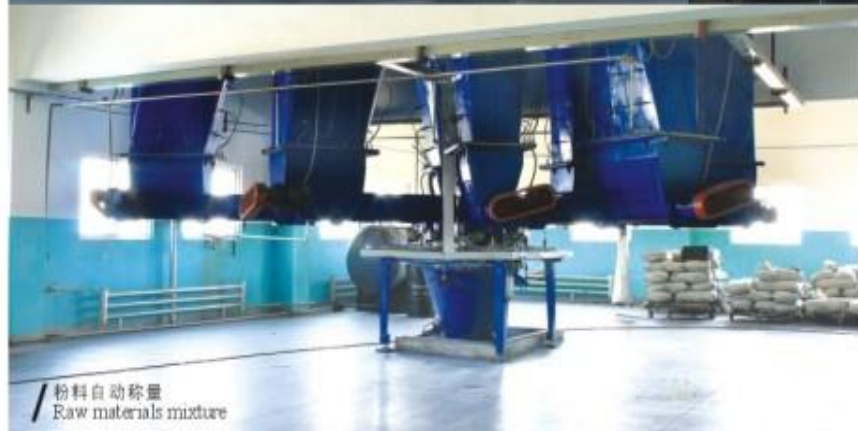
/ 粉料储料罐 Raw material tank
