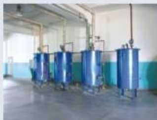
11 / 油料储料罐 Oil mixture equipment
